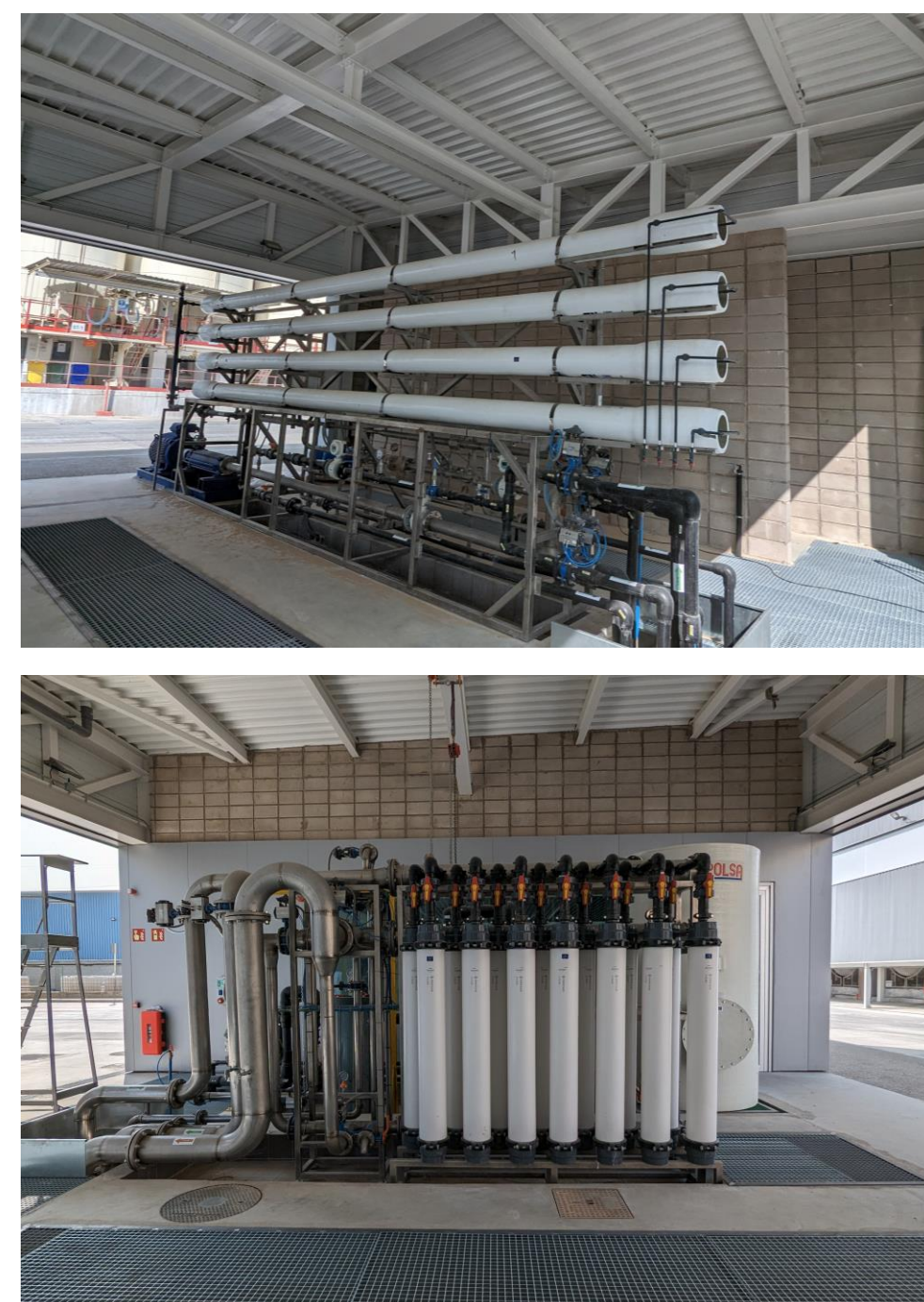
Figure 3. UF and RO pilot installations at IQE
